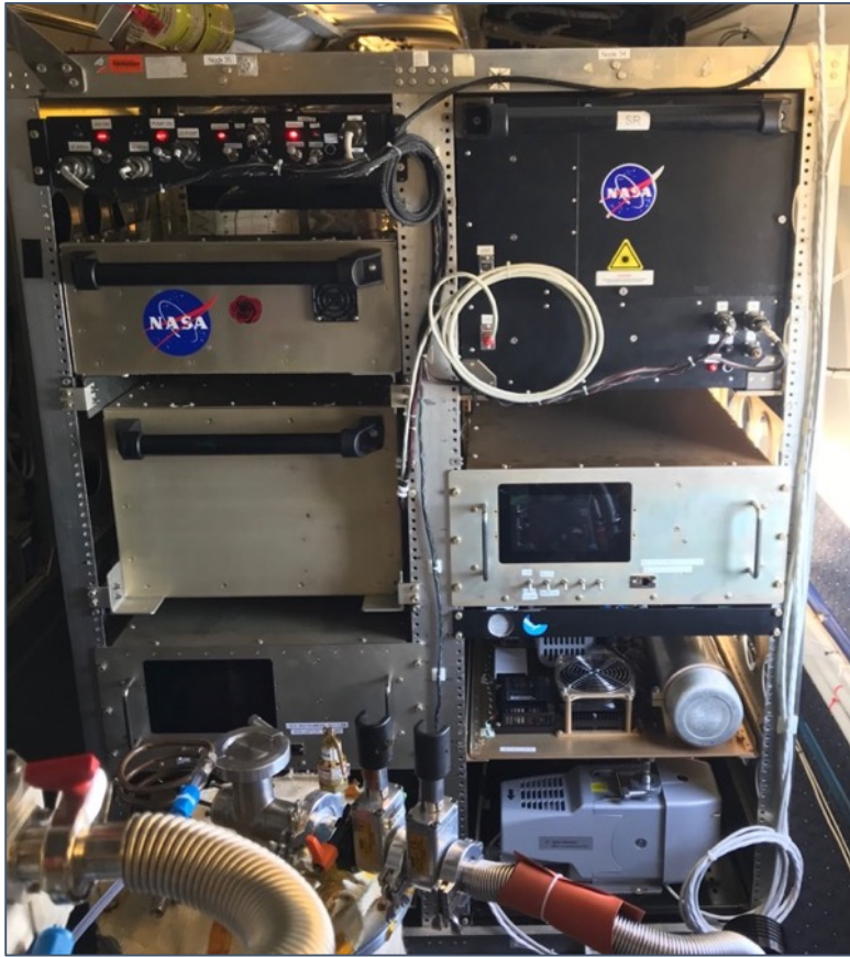
ROZE on DC-8 rack
